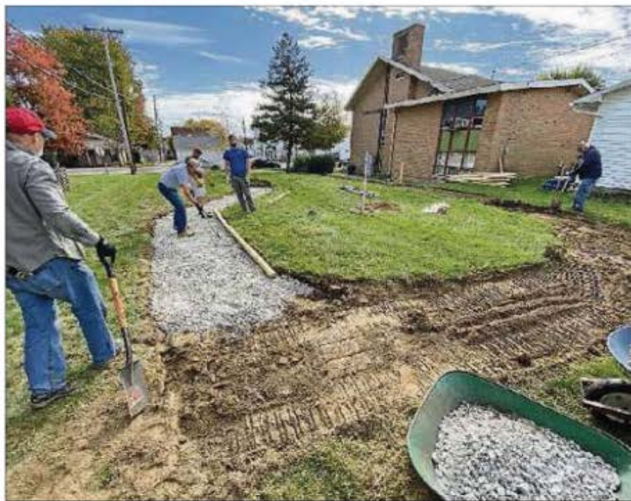
Volunteers work alongside Dave Wickham, the owner of the soon-to-be-opened Joy & Whimsy Depot in Lewisburg, constructing an outdoor prayer garden next to the former church building. CONTRIBUTED
